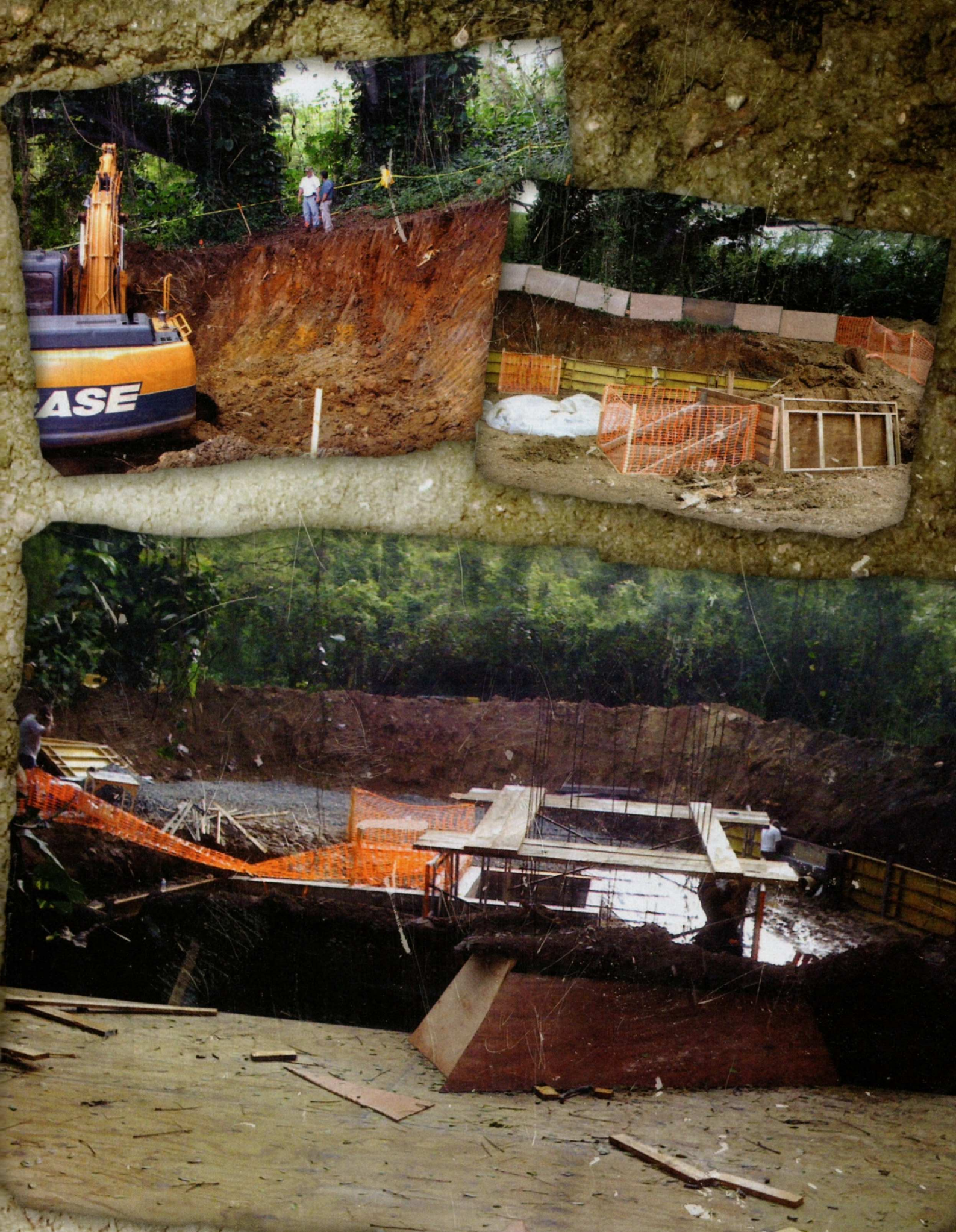
Above: The digging out of the Hawaiian landscape is a painstaking process: the team have to consider the way the ground will look after they've dug it away; the safety of the area for the cast and crew, and the huge array of structural devices that will not only maintain the Swan 'set's' appearance, but also be a workable environment for everyone on what is always an extremely tight shooting schedule.
